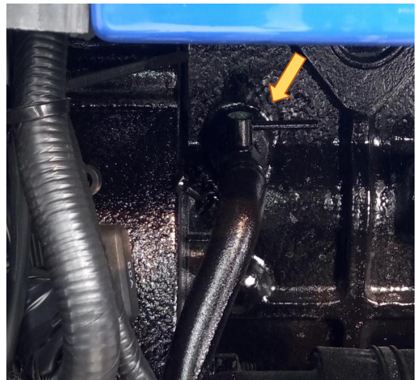
Water drain valve of cylinder
